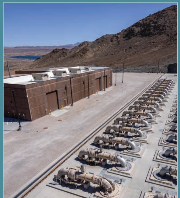
Low Lake Level Pumping Station
