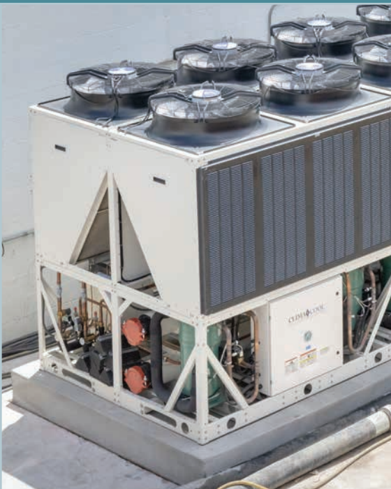
Dry-cooled evaporative cooling system
