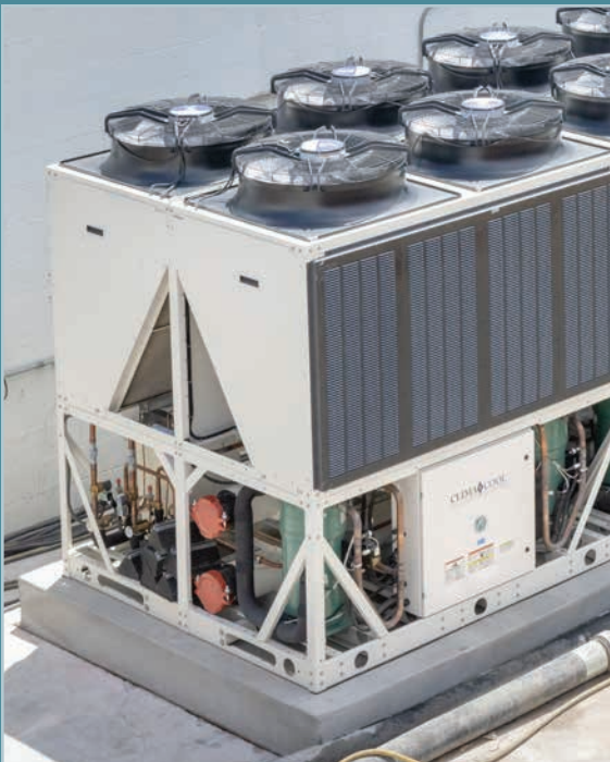
Dry-cooled evaporative cooling system
