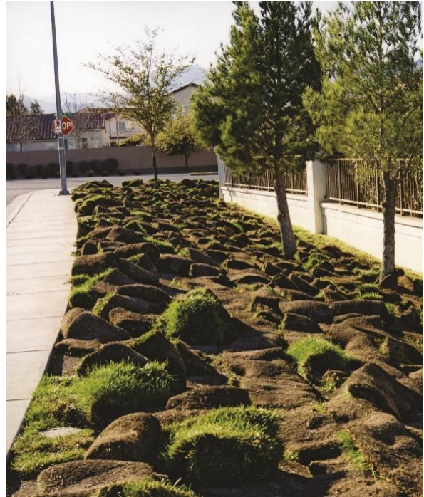
Photo: Streetscape turf. Replacing turf along streets and in medians will improve water efficiency and reduce water waste.
