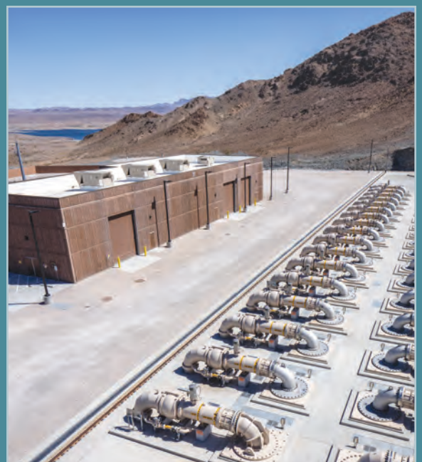
Low Lake Level Pumping Station
