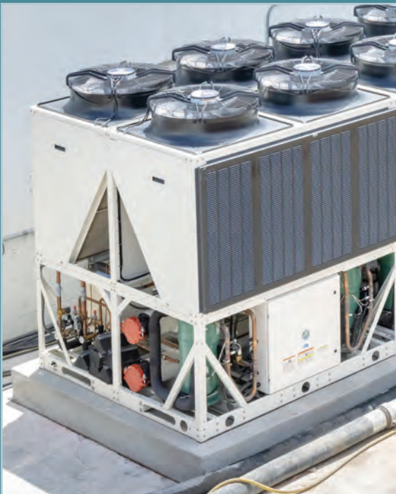
Dry-cooled evaporative cooling system
